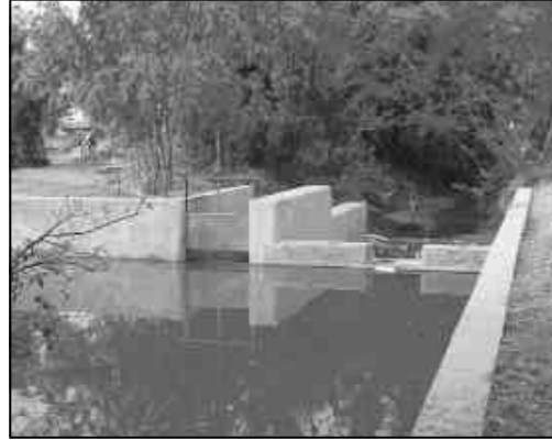
A dam constructed by the community people with support from RRN to provide irrigation facility to their farmlands.
