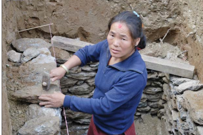
Women are increasingly taking up skilled jobs: a women constructing reservoir tank (Dhupu, Sankhuwasabha)
