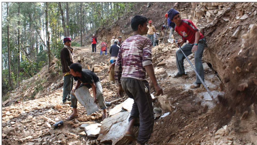
Local people participating in rural agriculture road construction in Naumule VDC, Dailekh
